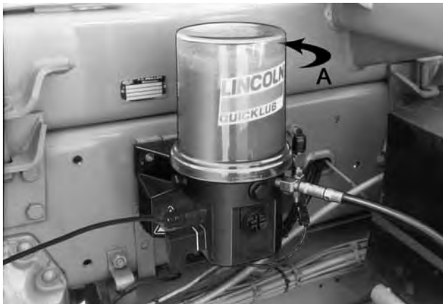
Fig. 9-1 Fill pump reservoir
